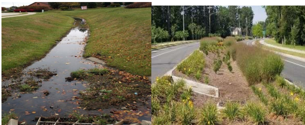
Fig 1: A Natural drainage ditch (SOURCE: Aquabrightllc.com Source: www.google.com .)
