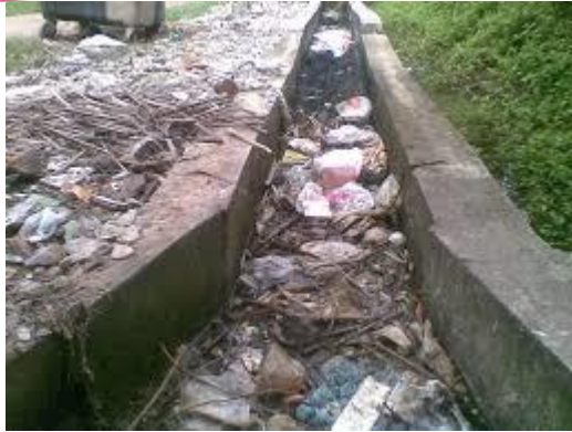
Fig 4 (a) Blocked Drains
